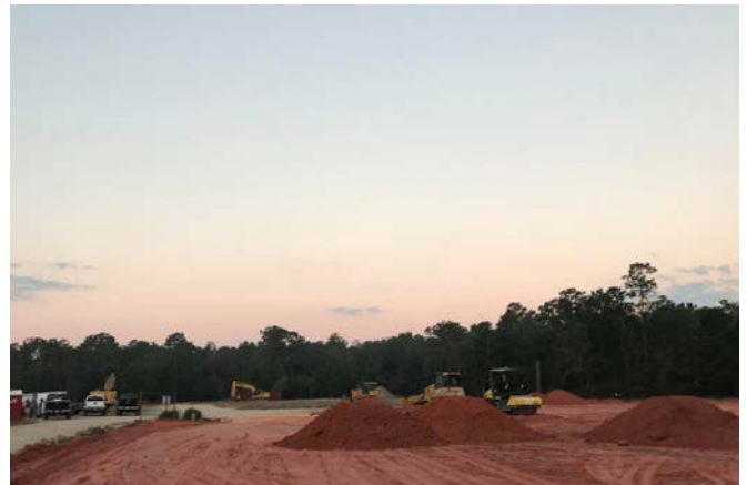
January 2023: Site clearing for the new STHS Surgery Center on Bootlegger Road.
